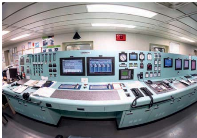
Everything at a glance – the effect of digitalisation is clearly visible in ship control centres. Cloud connectivity provides new opportunities for networking in the shipping industry. Source: WAGO
