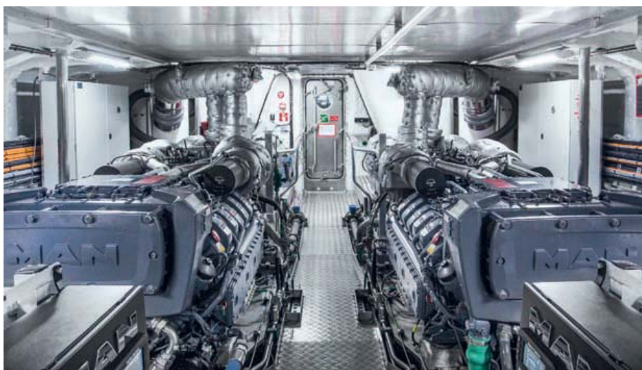
View of the engine room of the Luna with the twin MAN D2862 12-cylinder engines, each rated 1,029 kW in terms of power at 2,100 rpm Source: MAN Engines/Andrew Chin
